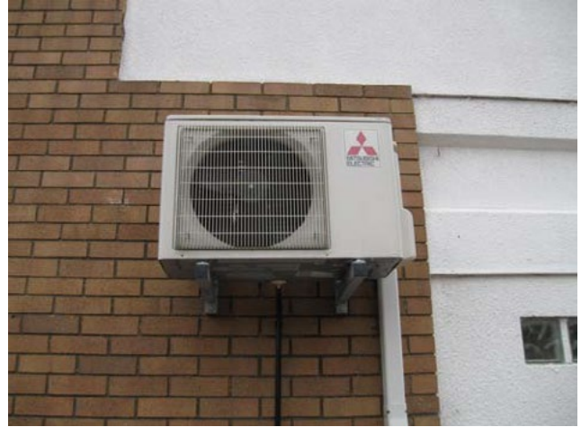
Outdoor ASHP Unit
