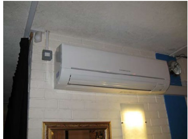
Indoor ASHP Unit
