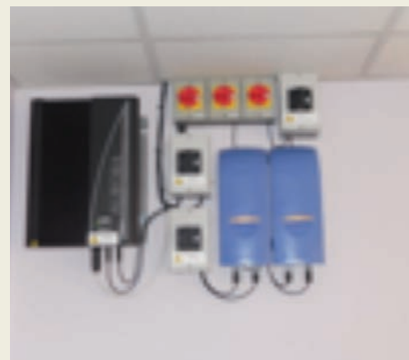
Air source heat pump at Bedford Rural Communities Charity
