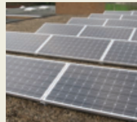
Solar PV panes installed on Scott Lower school's roof.
