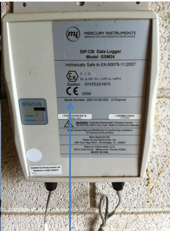
This logger is an Energy Assets data logger installed by Energy Assets on behalf of British Gas
