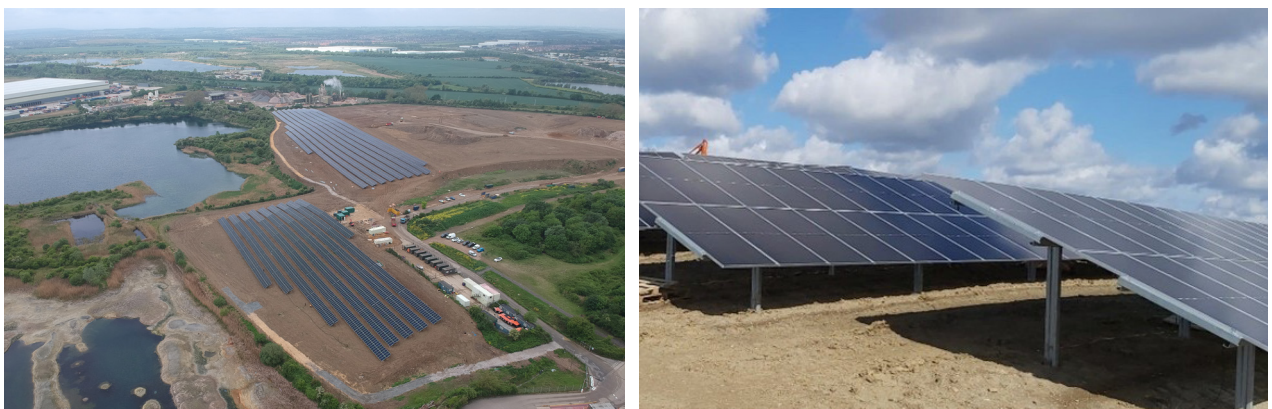
Photo: Birds Eye View of Elstow Solar Farm and close-up of solar PV installed.
