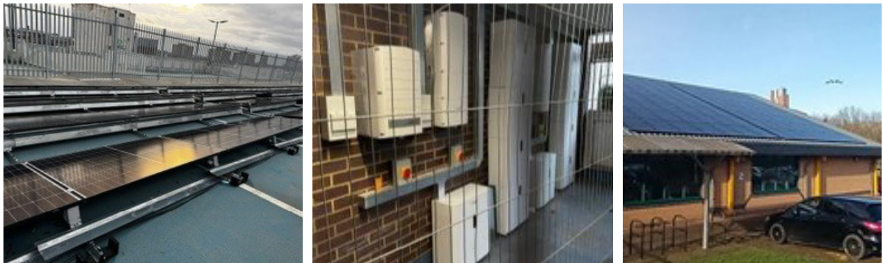
Photos: Brand new solar panels and battery storage installed at Queen Street Car Park (left and centre); Solar panels installed at Kempston Swimming Pool (right).
