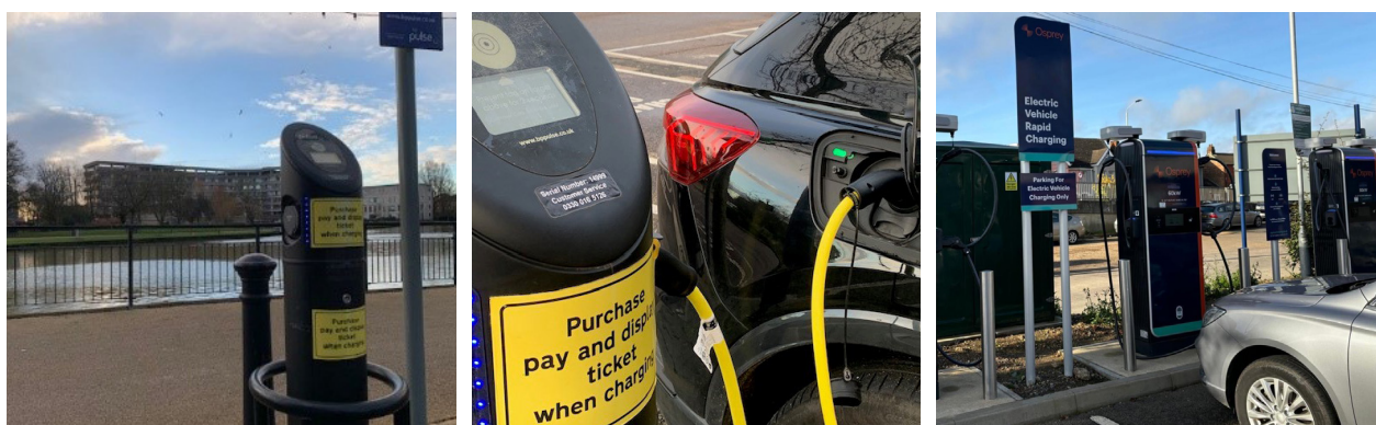
Photos: EV Car charging in Riverside Car Park (left and middle), EV Chargers in Rope Walk Car Park (middle).
