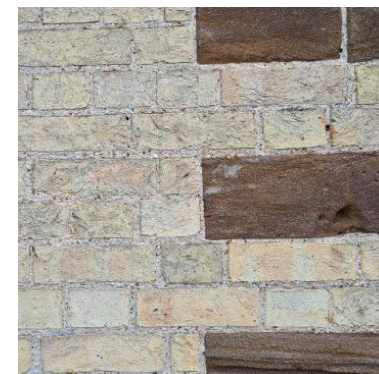
Figure 19 Ironstone quoins with surrounding buff brick bedded in tight lime mortar joints.
