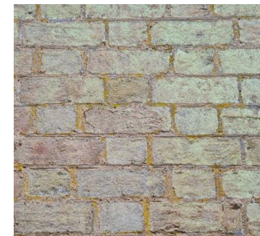
Figure 14 Buff brickwork laid out in Flemish bond with ruled joints at the New Manor House. The same treatment is used for the stables.
