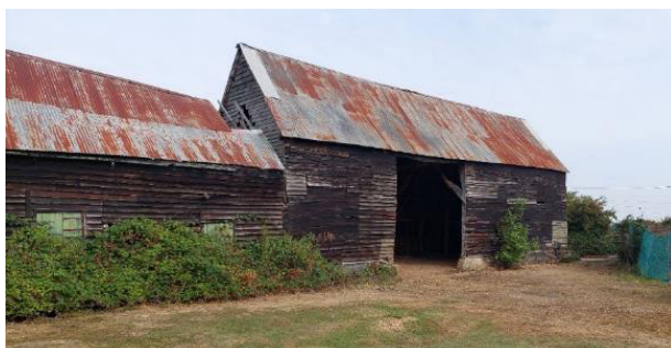
Figure 13 The grade II listed barn at Lower Farm, which is aisled to the rear side. A later extension leads off the southwest gable end.
