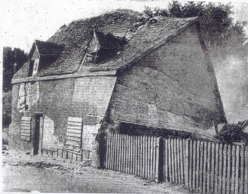
The cottage at Elstow which has taken a lot of knocks from traffic in past years.
